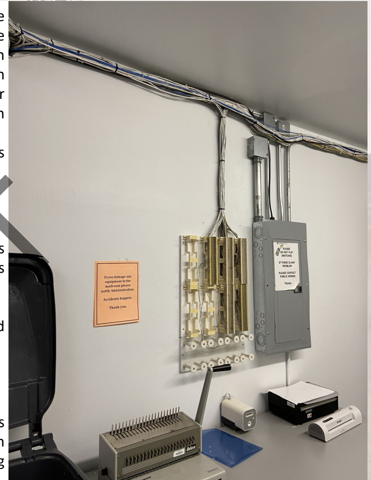
Figure 8-3. Exposed wiring in City Hall
