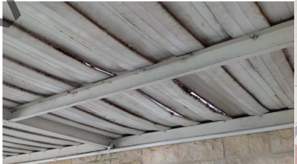
Figure 8-1. The Canopy around the Golf Course Club House. You can see the deterioration and damage that has happened due to weathering.
